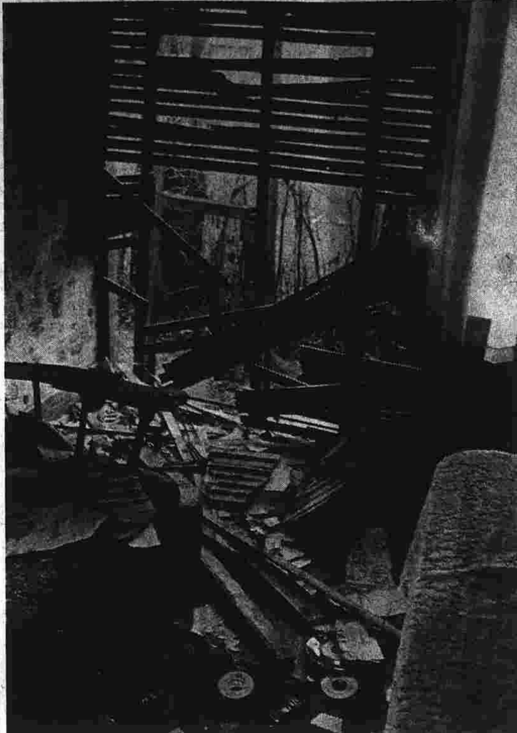
Lightning Caused This Hole in the Side of the Kelly House
